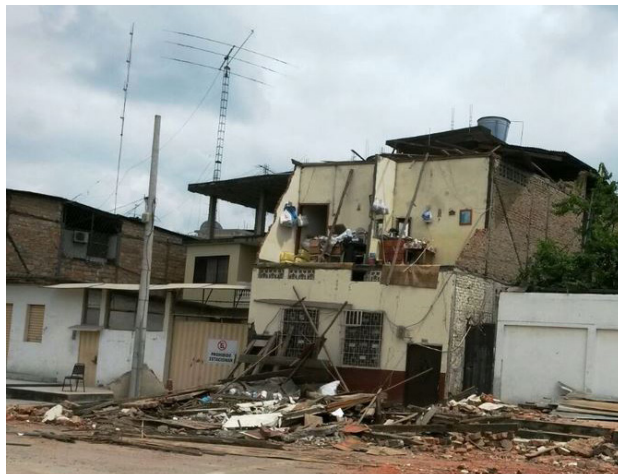
The destroyed home of well-known Ecuadorean DXer Lilian de Ayala, HC4L. She barely escaped when her house collapsed. Although her shack was destroyed, both of her antennas survived.
