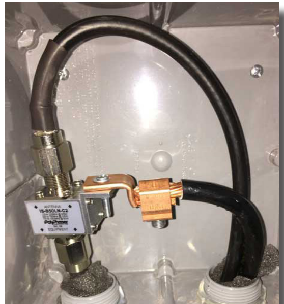
Lightning Arrestors: The last line of defense
