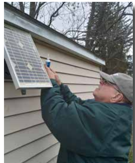
Steve finishes the solar panel install by weatherproofing the wiring pass thru into the shed
