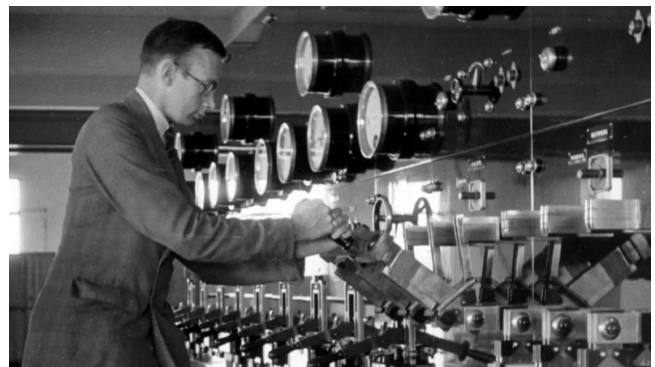
Changing the Feeder Switch at Droitwich Transmitting Station, October 1935. Long wave transmissions from Droitwich started in 1934
